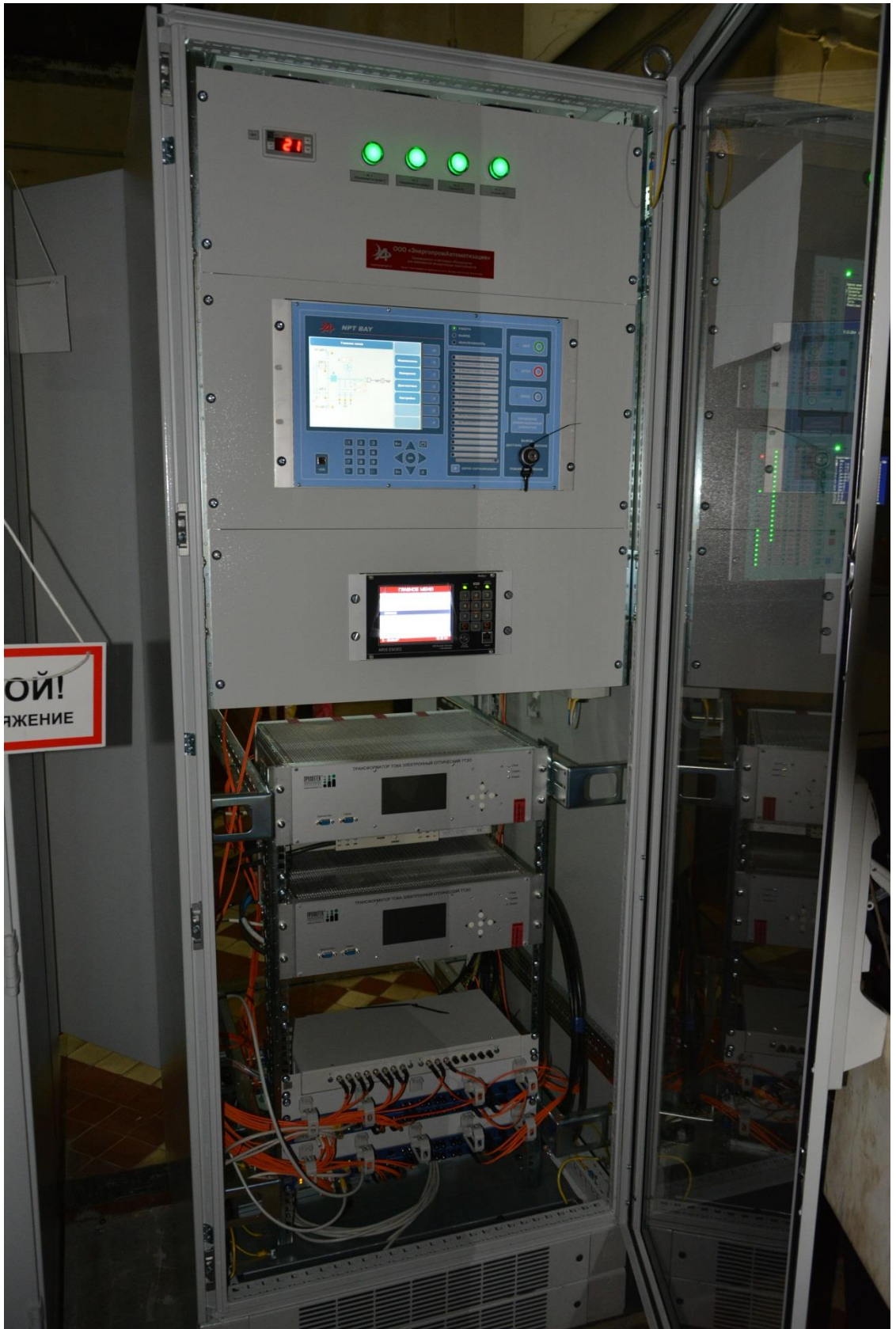
Figure 5 – Cabinet of bay controllers
