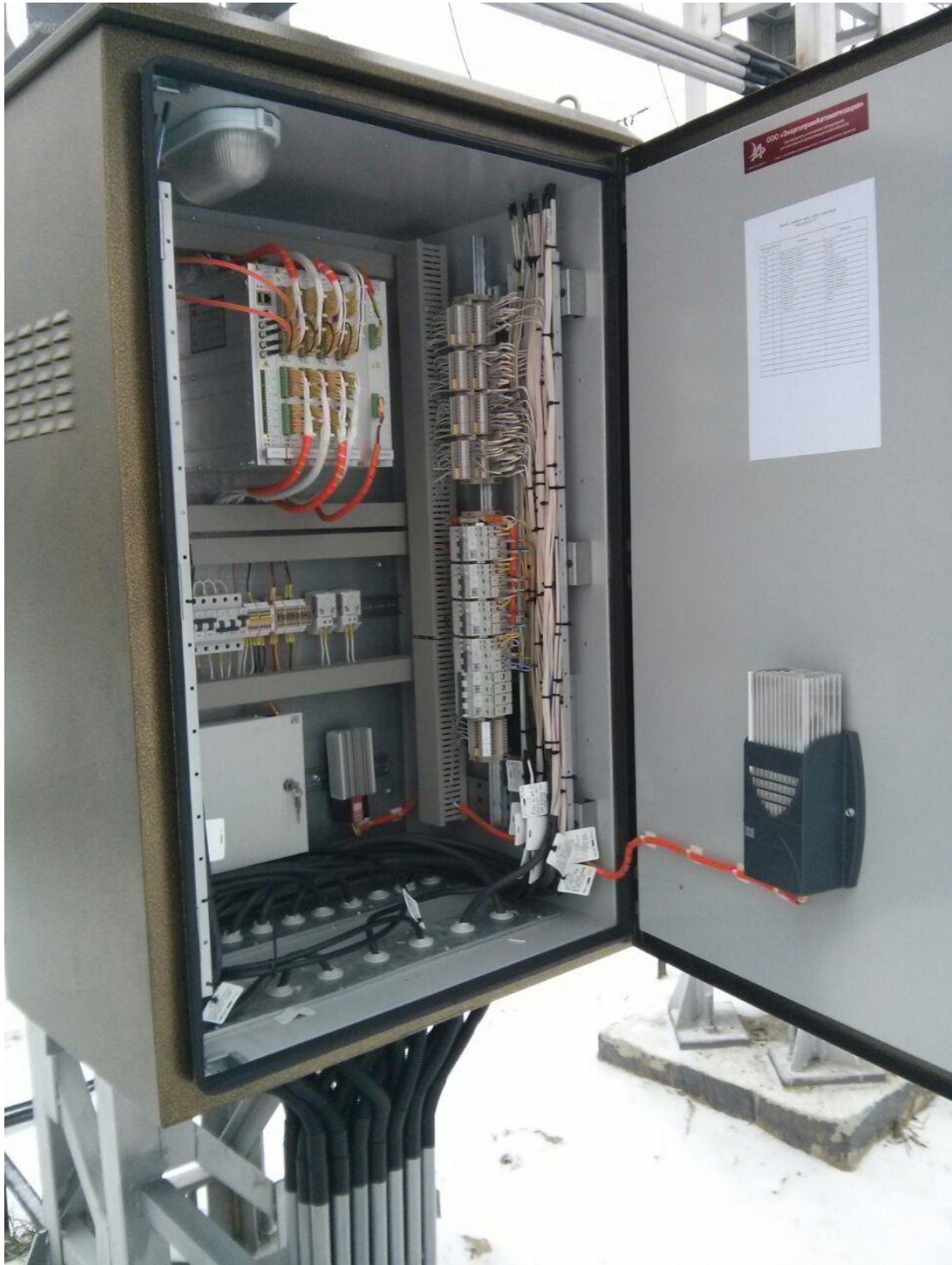
Figure 4 – Cabinet of RTU
