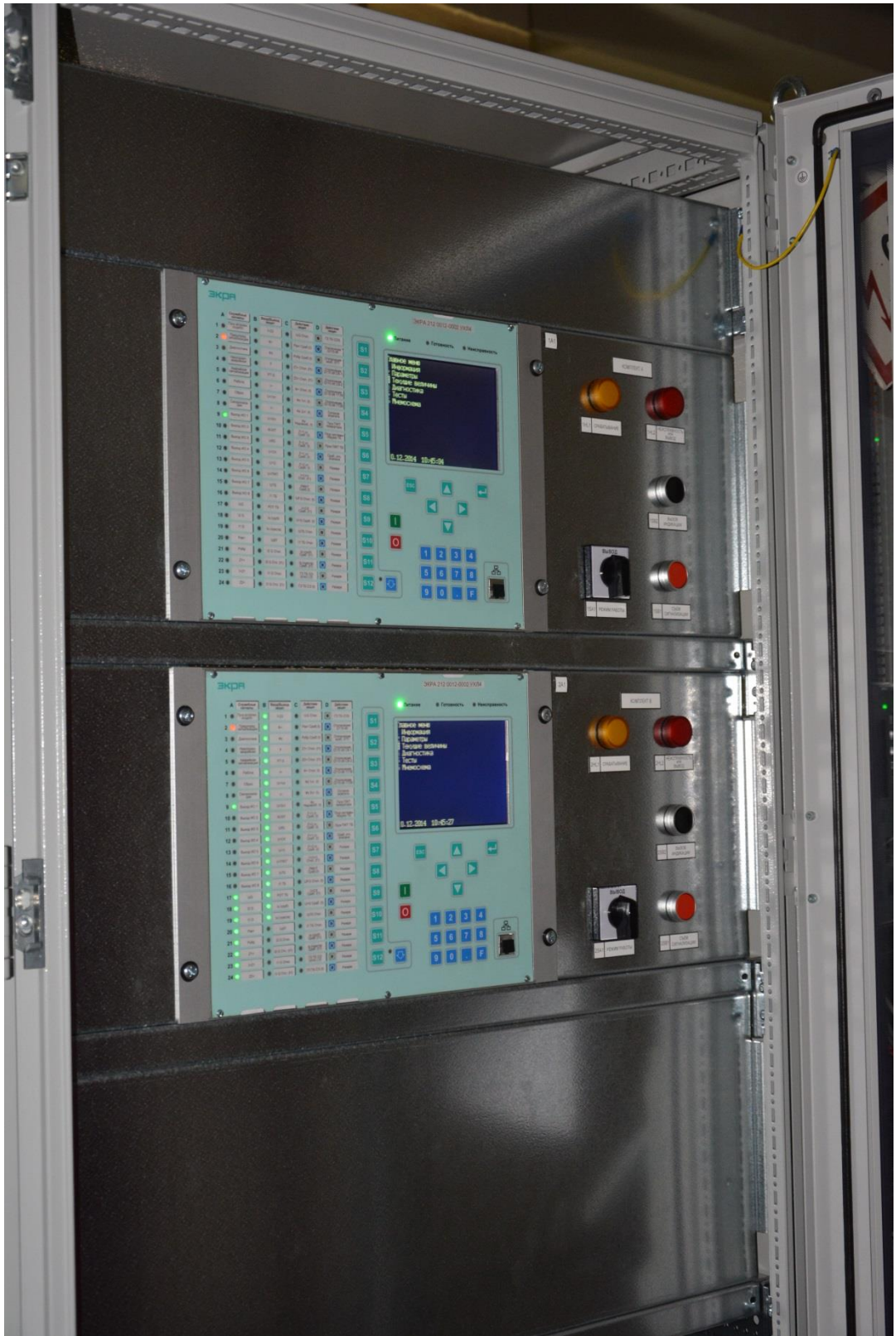
Figure 6 – Cabinet of relay protection EKRA 200
